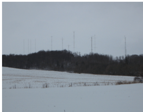
The antenna "farm"
